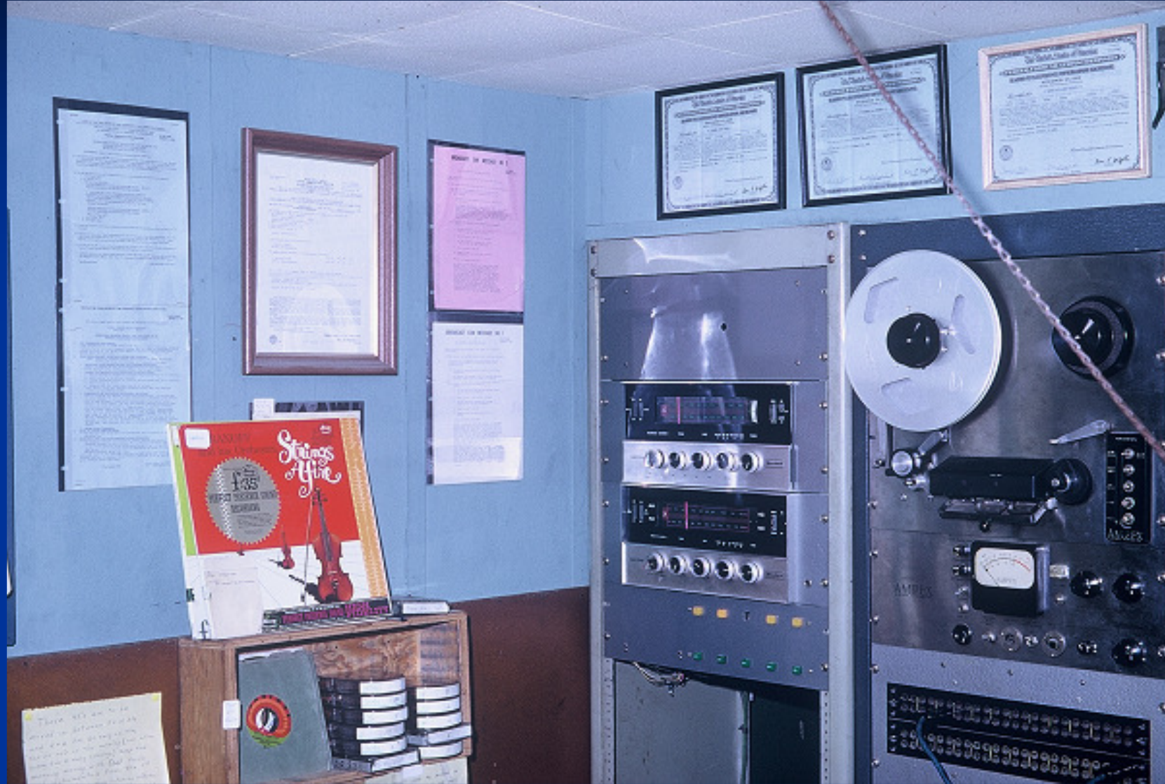
Station licenses and equipment racks in the Eames Hall Studios. Except for the console, the equipment shown was the total equipment inventory.
